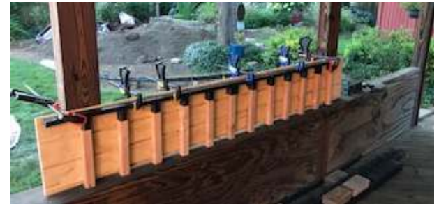
Jig construction of an 8ft section of ladder base for track bed. (T&L Dove)
